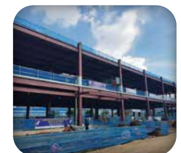
HANA MICRON Investor/main contractor: Sungdo ENG Vietnam Co., Ltd Address: Van Trung IP Bac Giang
