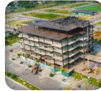
VAN DON URBAN AREA Investor/main contractor: Phuong Dong JSC Address: Van Don, Quang Ninh
